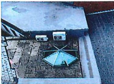
Aircon slab leaking
