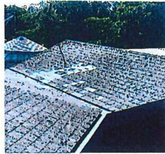
Tiles remedial work required
