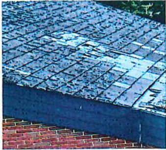
Tiles damaged and dislodged
